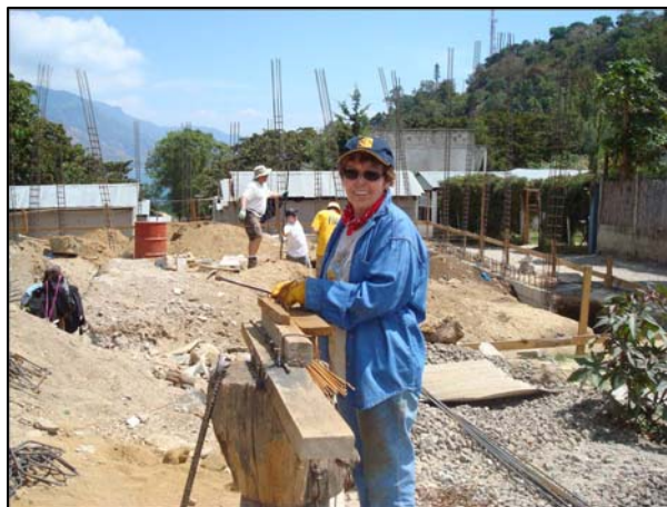
LaVonne Bullinger works with rebar at the First Response Station in Guatemala.
